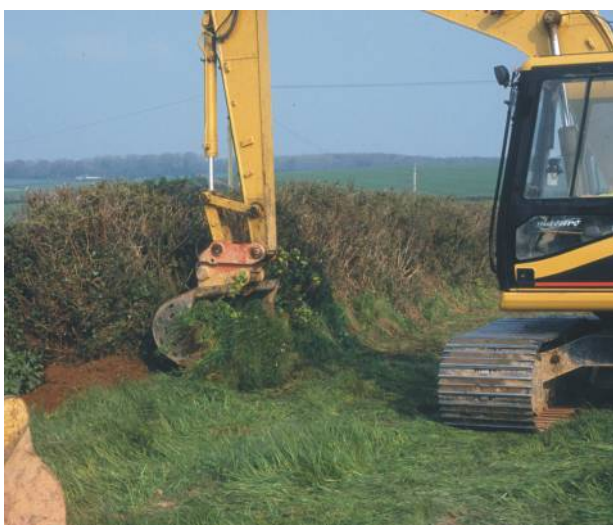
Figure 2: Remove slumped soil and turf from the base of the hedge, on the side facing the direction of movement. ©Peter Chamberlain
