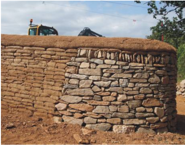
This high steep bank has been carefully restored as part of the South West reinforcement gas pipeline to match the original. Note the innovative use of hessian sacks filled with topsoil to build up the steep sides and hessian textile to stabilise the top. The original hedgebank shrubs have since been replanted successfully. ©Laing O'Rourke
