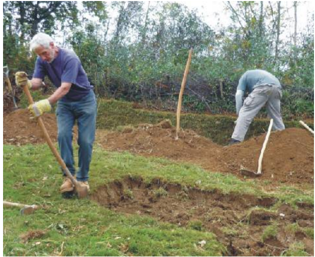
Don Gaskins cutting turves to re-face the bank behind. Note the curved handle of the Devon shovel, useful as a form for the concave face of the bank. ©Maxine McAdams
