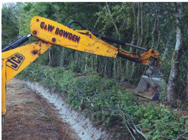
Repairing a damaged bank using a wheeled digger. The hedge has been steeped along one comb, leaving the other side to do later. ©Robert Wolton
