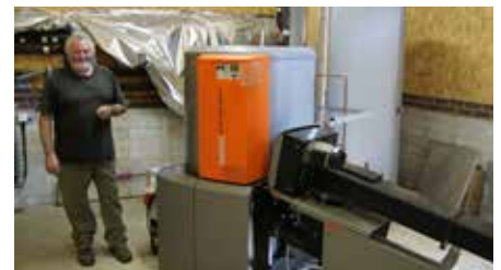
Woodchip boiler used to heat a Devon farmhouse
