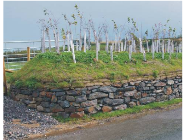
Figure 7: This rebuilt section of Devon hedge with stone and turf facing closely matches the profile and shrub mix of the original. It was reinstated following installation of the South West reinforcement gas pipeline. ©Laing O'Rourke
