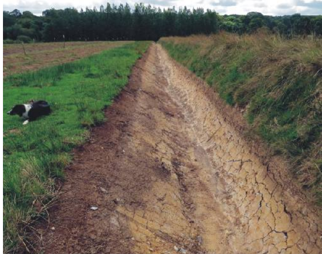
Figure 2: The new bank on the right has been built and turf faced using an excavator. The ditch provided most of the material for the bank. This bank will soon be planted with shrubs and trees. ©Robert Wolton
