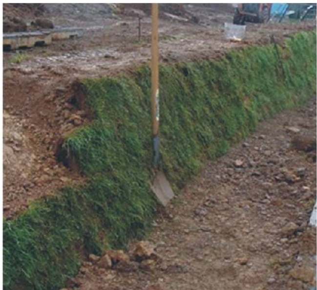
Figure 3: Construction of a turf faced bank showing the progressive coursing of turves and build-up of fill. ©Paul Couttie
