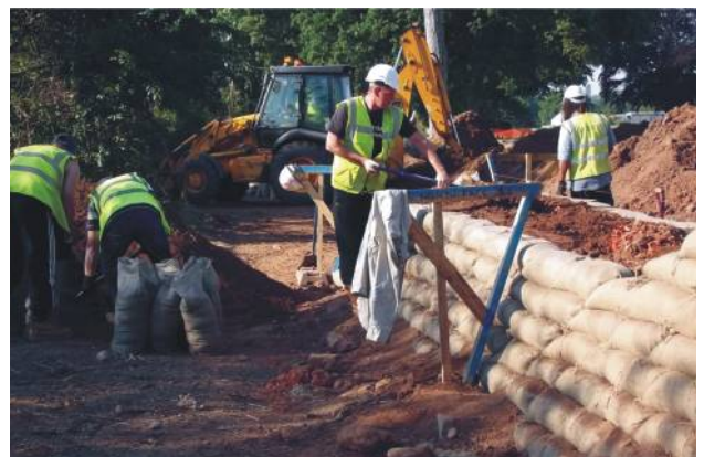
Figure 4: Hessian sacks being used to construct a bank on the Exe Estuary Trail. Note that both machinery and hand tools are used. Shape formers (painted blue) were used to guide the profile, line and level of the bank during construction. ©Paul Couttie
